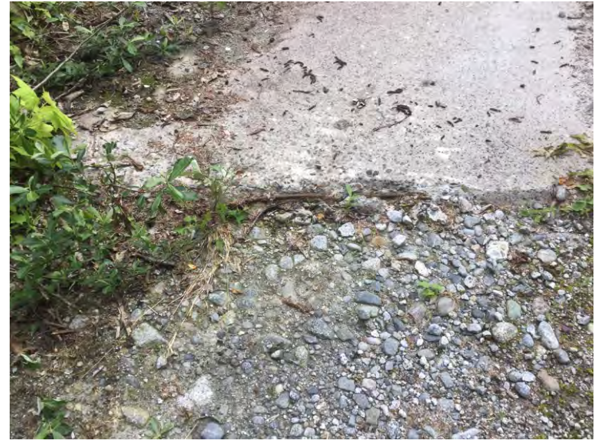
Deck damage at left approach
